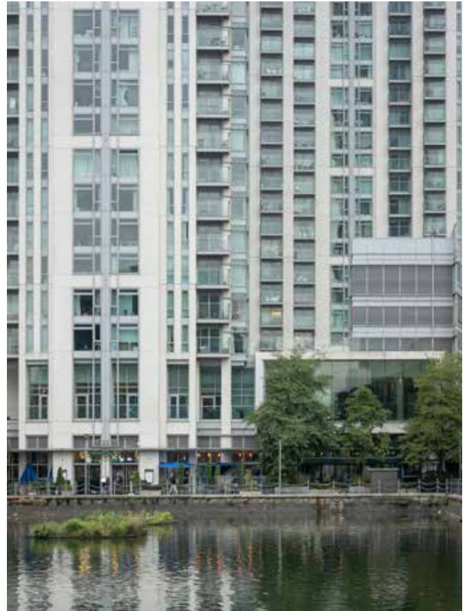
Full ceiling height windows are at risk of overheating in summer and heat loss in winter.
