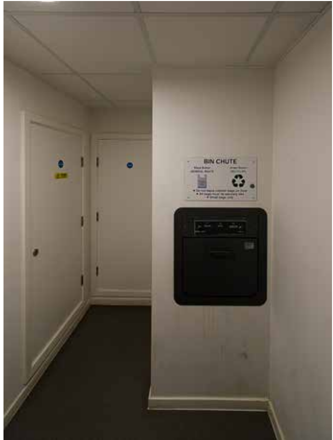
An ineffective waste chute. It is not located in a special room, signage is unclear, the area lacks ventilation and the surrounding area would be easily damaged if waste was left on the floor.
